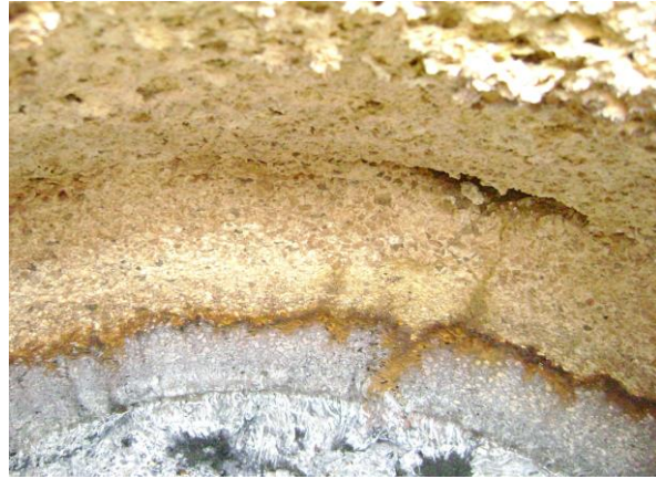
Figure 2: Concrete damaged and crumbling due to MIC
